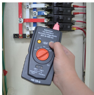
Detect voltage in circuit breaker
